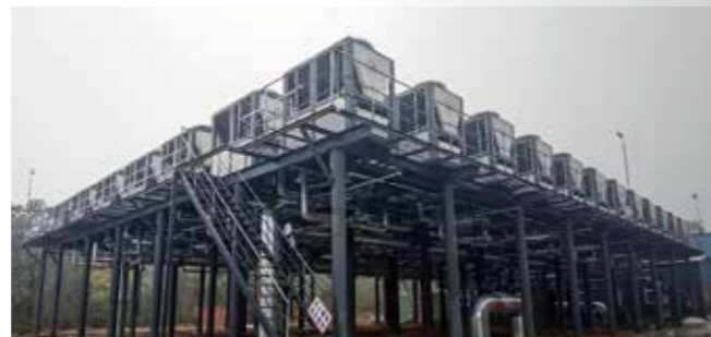
Baizhai Town, Xinmi City, Henan Province Heating Area: 600, 000m 2 Heat Pump: 150kW/unit Total: 130Units
